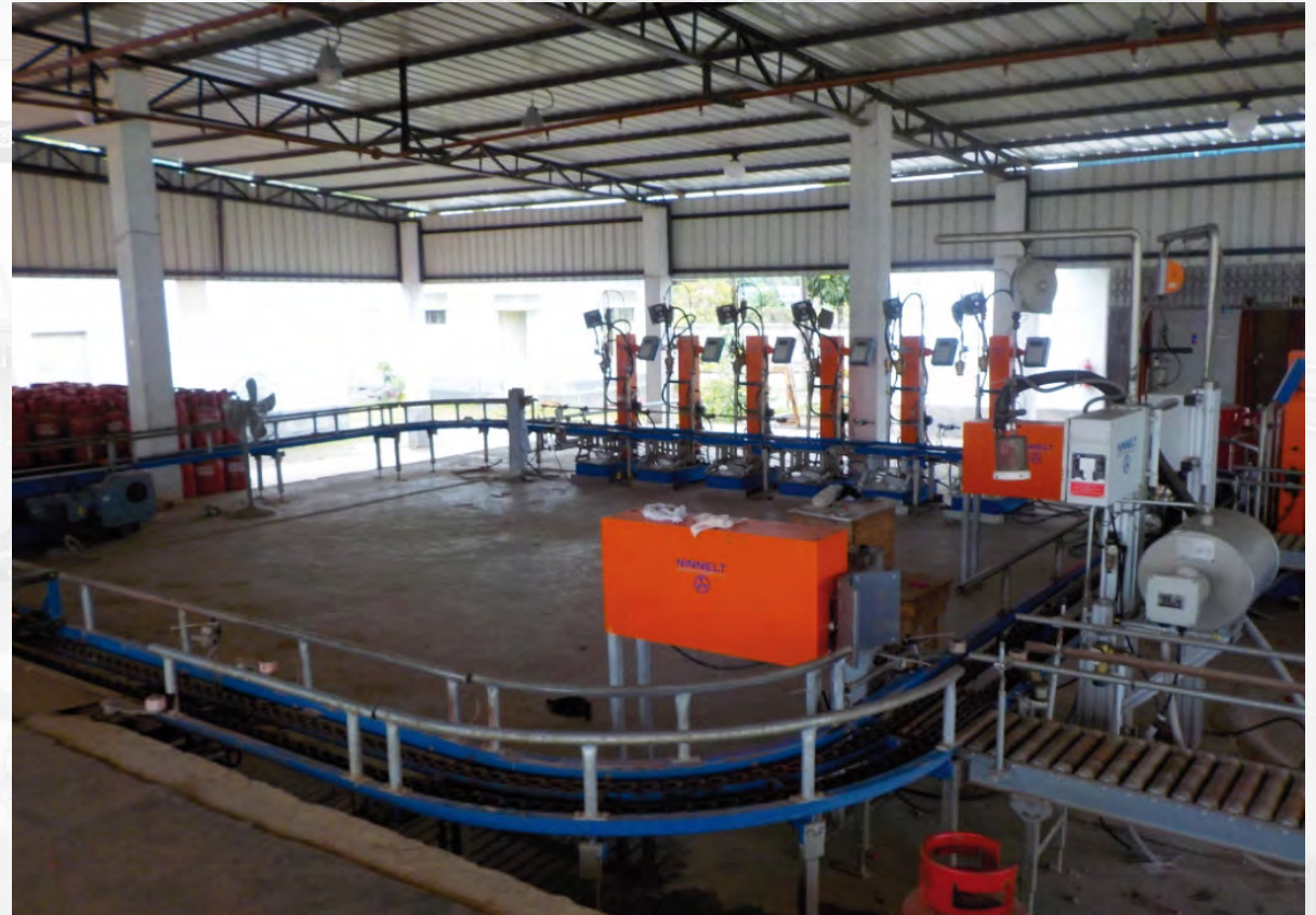
Inline Filling Station
